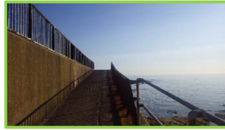
Access ramp cracking and hand railings damage (/4601c10).
