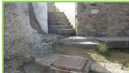
Minor erosion of concrete and undermining of steps on island (/4501c03).
