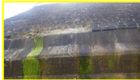
Sections of brickwork missing at south end of upper sloping masonry wall (/4601c06).
