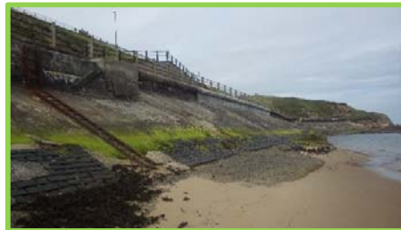
Major spalling and cracking, abrasion and exposure of reinforcement at toe. New section of coping stone (/4701c27).
