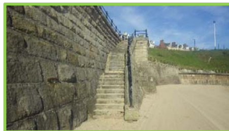
Concrete repairs required at base of the steps in bay (/4701c13).
