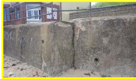
Wall south of Boardwalk Cafe, spalling and exposed reinforcement mesh (/4501c09).
