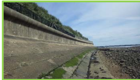
Abrasion to concrete toe of concrete recurved wall (/4801c07).
