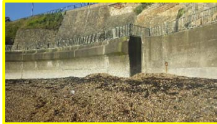
Railings poor and abrasion to lower section of concrete wall (/4701c01).
