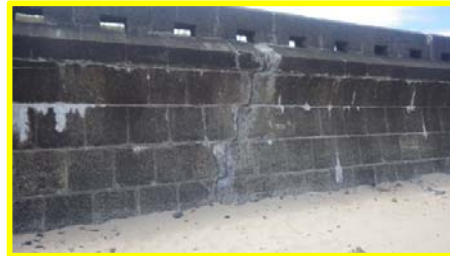
Diagonal cracking through blocks south side of Rendezvous café (/4501c07).
