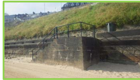
Cracking to concrete on access steps, handrails repaired (/4701c23).
