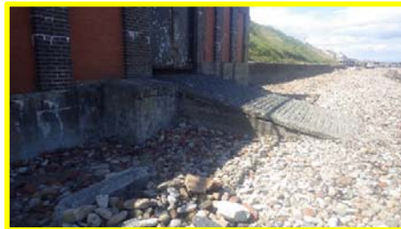
Cracks and gaps beneath lower ramps (/4601c02).
