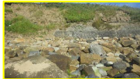
Evidence of slumping (/4701c16).
