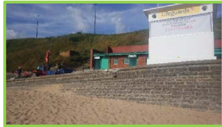
Damage to coping stones (/4701c018).
