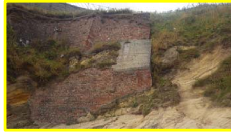
Missing mortar and gaps in upper wall (/4701c10).
