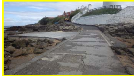
Cracks and patch repairs in causeway to St. Mary's Island and new concrete turning head (4401c25)
