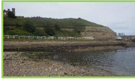
Revetment in Priors Haven in good condition, vegetation at top of wall (/4801c02).
