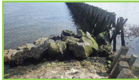
Stone protection at end of jetty in good condition (/4801c10).
