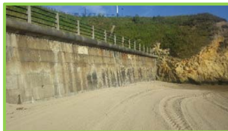
Walls in the southern section of the bay in good condition and level of sand good (/4701c12).
