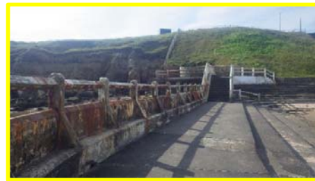
Interior of top wall spalling and staining (/4701c24).
