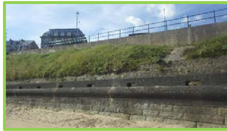
Missing mortar to joints and coping stones (/4701c23).
