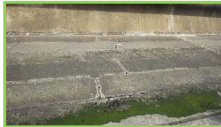
Cracks in revetment and gaps between panels (/4801c07).
