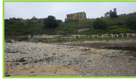
Masonry revetment in good condition, vegetation at the top of wall (/4801c02).
