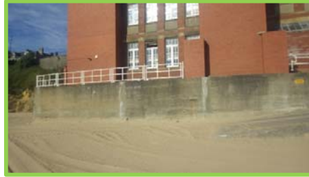
Concrete protection to Dove Marine Laboratory in good condition. Joint repairs carried out (/4701c09).
