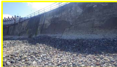
Severe spalling and cracking along straight section of wall (/4601c03).
