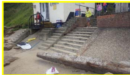
Undermining of steps to Lifeguard Centre King Edward's Bay (/4701c28).
