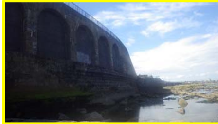
Missing mortar and gaps beneath long sections of copings (/4601c08).
