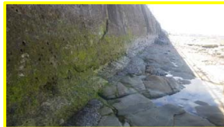
Severe spalling and cracking of rendering (/4601c03).
