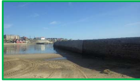
South Pier in very good condition following reconstruction. Beach levels good (/4701c15).
