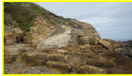
Considerable abrasion and damage to steps (/4701c26).
