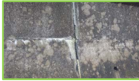
Trinity Road sea wall spalling of some joints (/4501c04).
