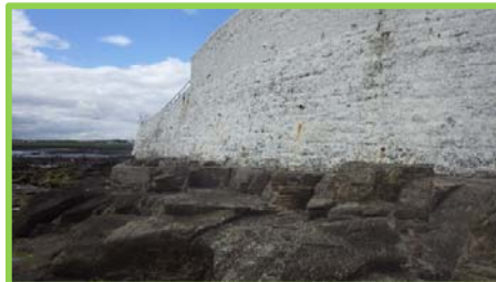
Walls on west of St Marys Island well founded and in good condition (/4501c03).
