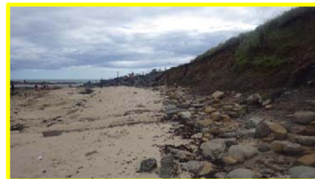
Evidence of slip adjacent to rock armour defences north of St. Mary's Lighthouse (/4401c24)
