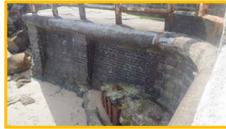
Wall at southern landward tie in of pool with apron undermined (/4701c25).
