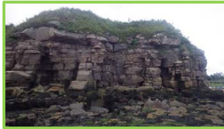
Fractured rock at Freestone Point (/4801c11).
