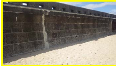
Some construction joints filled, others require attention, coping stones have missing mortar (/4501c07).
