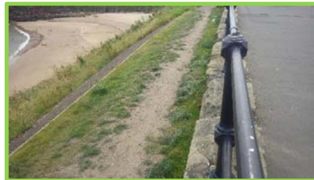
Section of upper slope top soiled and seeded since 2012 when cracking was visible in bitmac footpath (/4701c27).
