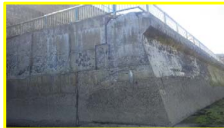
Missing section of concrete, undermining railing post, vertical and horizontal cracking (/4601c07).
