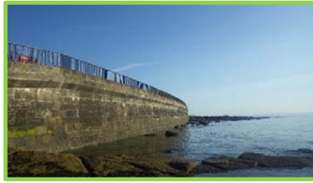
Cracks, joint gaps and abrasion around joint gaps increasing at south end (/4601c10).
