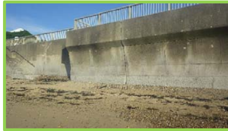
Concrete wall in good condition, abrasion to lower section of wall (/4701c01).
