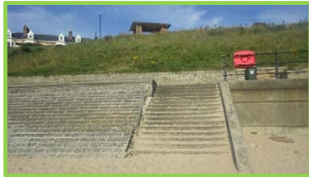
Localised damage to steps and crest of masonry revetment with gaps in joints leading to cracking (/4701c019).
