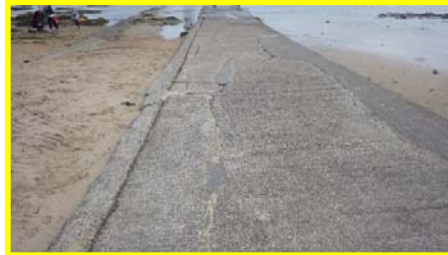
Cracks in causeway to St. Mary's Island (/4401c25).
