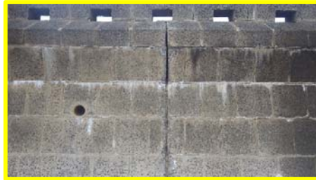
Further repairs to joints required in Whitley Links sea wall (/4501c07).
