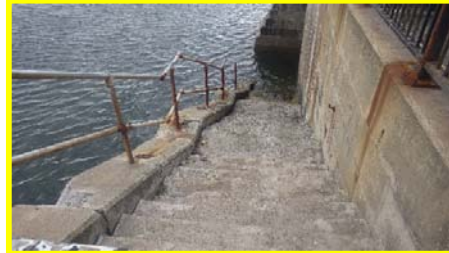
Damage to base of steps and handrailing (/4701c06).
