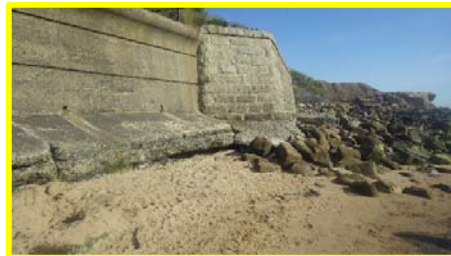
Erosion undermining the concrete toe apron, no change since 2012 (/4701c17).
