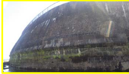
Heavy staining in places, evidence of erosion at the base and horizontal gap in upper brickwork (/4601c04).
