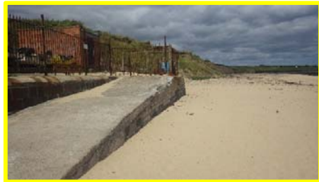
Concrete ramp boathouse in reasonable condition minor spalling (/4501c05).
