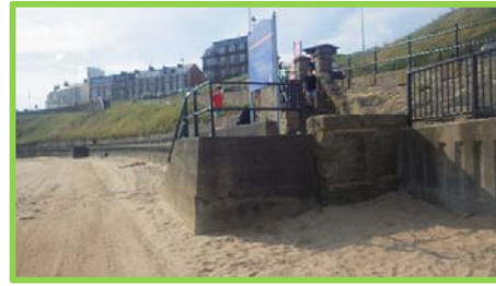
Cracking to access steps similar to 2012 (/4701c22).
