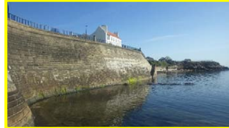
Minor joint repairs required. Some undermining of the concrete apron, (/4701c06).
