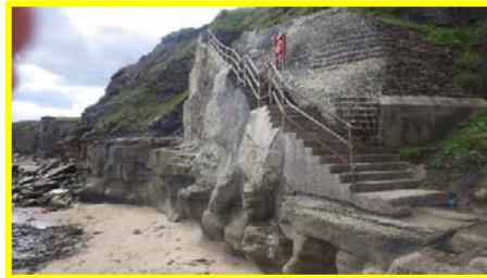
Old Hartley Steps retaining wall and hand rail in fair condition (/4401c23).
