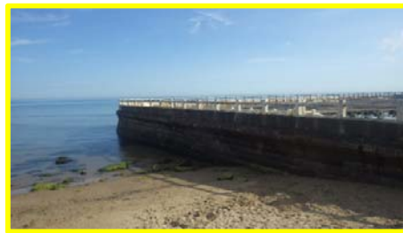
Tynemouth Pool abrasion and spalling on wave return wall (/4701c24).
