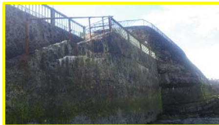
Steps in very poor condition, horizontal and vertical cracks (/4601c07)
