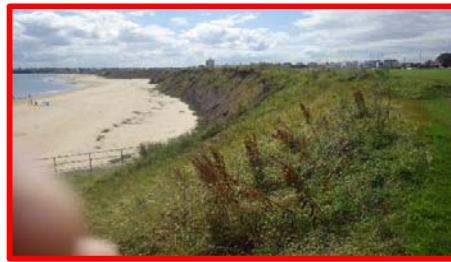
Slumping of cliffs at end of Whitley Sands adjacent to golf course (/4501c05).
