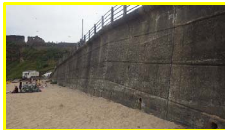
Concrete wall in King Edward's Bay in good condition, also railings (/4701c28).
