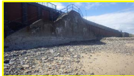
Abrasion and cracking to access steps (/4601c02).
