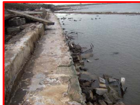
Severe damage to promenade and loss of coping stones, surfacing and railings at south end (/4601c08).
