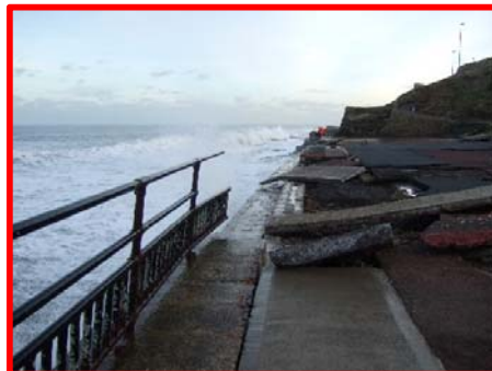
Severe damage to promenade and loss of coping stones, surfacing and railings at south end (/4601c08).
